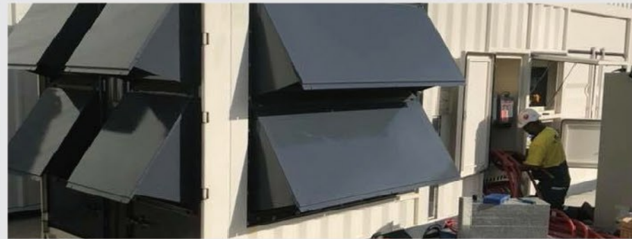
↑ Airport backup generator
