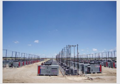
Botswana 70MW diesel power plant ↑
