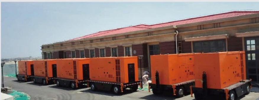
← Harbour project with trailer mobile Stage III genset
